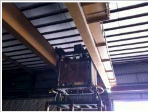
Bridge Crane after modernization
